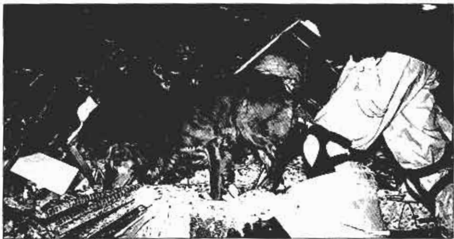
(Top) Rescue workers ascend the demolished structure in a man-basket to remove "widow makers"—chunks of concrete suspended from rebar. (Middle) Night work was challenging due to limited lighting and erratic weather conditions. (Bottom) Numerous canines were employed in the search. Due to the frequency with which they alerted to dead bodies, they became depressed. Firefighters substituted as live "victims" in the pile to cheer up and motivate the dogs.
