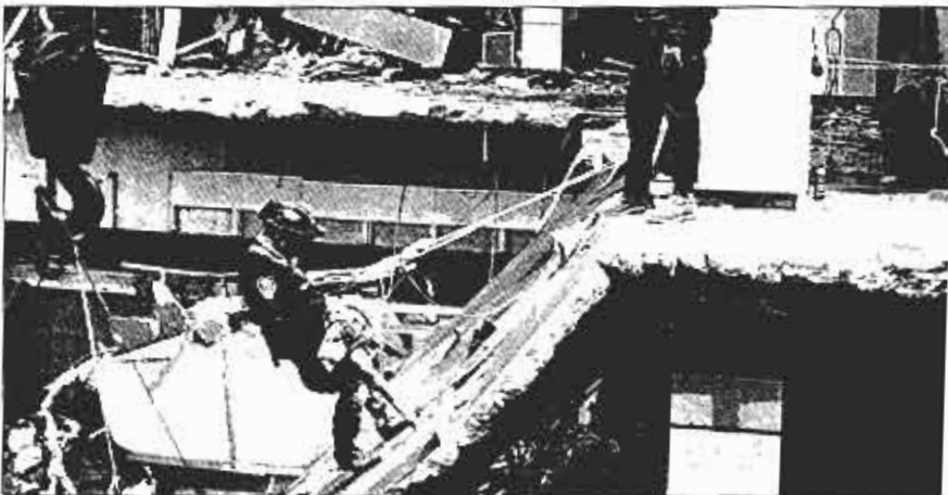
Cutting operation on a fallen slab. All operations were performed within the strictest margins of personnel safety possible.
