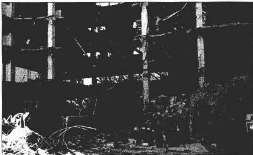
A trackhoe clears out “the Bowl” area (late in the incident). Note that the two columns to the right of the Bowl (F20 and F22) were left with no lateral support—the support had to come from prefabricated horizontal pipe shoring and steel banding. (Photo courtesy of Oklahoma City Fire Department.)
